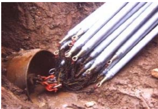
Above Left: A 36" backreamer was used to pull the 30 sticks of Bore-Gard through the bore.
